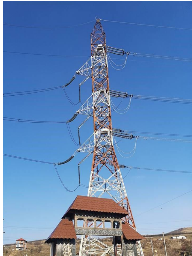
Photo: The 400/110/10 kV Cluj Est transformer substation
