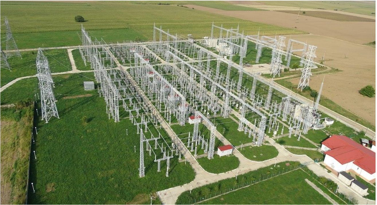
Photo: Gutinas 400/220/110 kV substation
