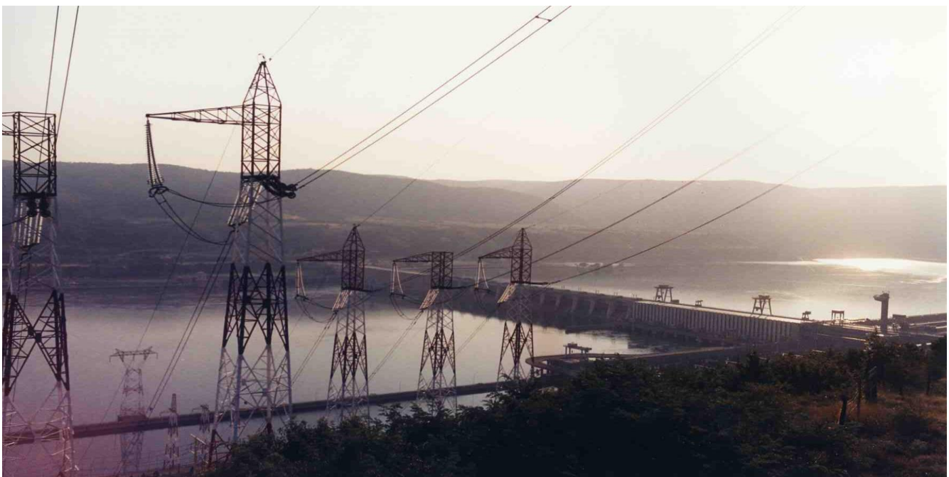
Photo: The first 400 kV slot of the National Power System - 400 kV overhead electric line, simple circuit, HPP Portile de Fier – Bucuresti Sud
