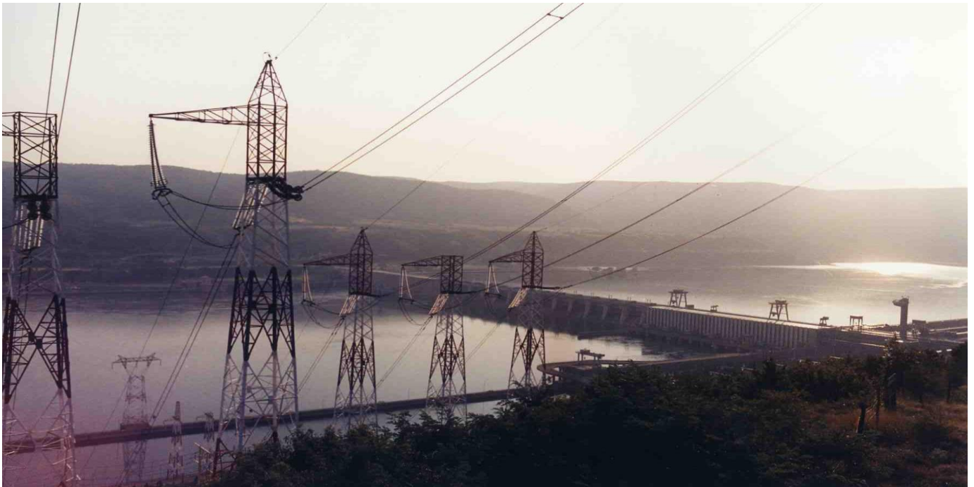
Photo: The first 400 kV slot of the National Power System - 400 kV overhead electric line, simple circuit, HPP Portile de Fier – Bucuresti Sud
