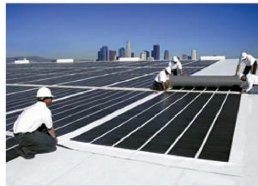
Flexible, Ruggedized Solar Sheet on Space-Constrained Commercial Rooftop
