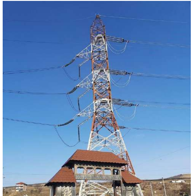
Photo: the 400/110/10 kV Cluj Est Transformer Power Station
