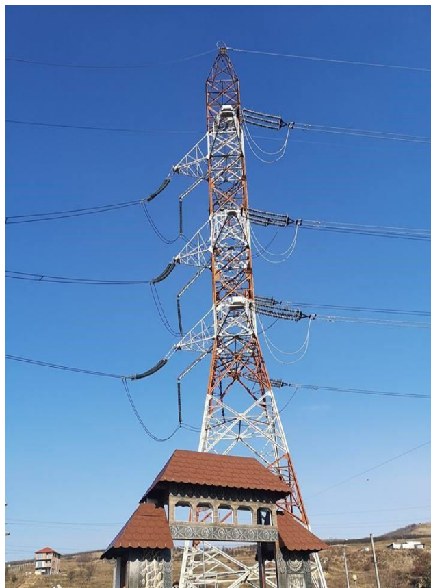
Photo: The 400/110/10 kV Cluj Est transformer substation
